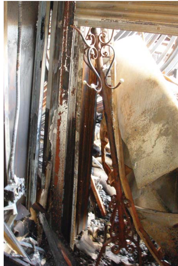
The closing path of rolling fire doors are required to be free of any objects that may interfere with door closing. Routine testing draws awareness to fire door locations and the need to keep their closing paths clear.
